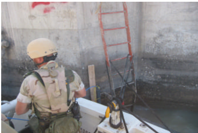
Figure 3. NAVOCEANO tide gage installation in Iraq.
